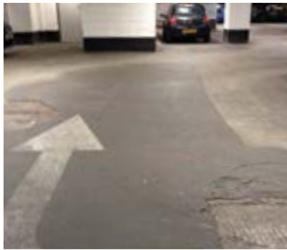
POOR QUALITY REPAIRS
